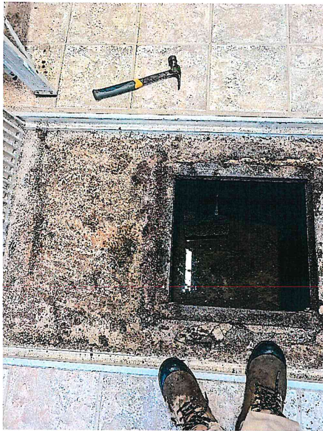
Rot in Concrete and Frame at Entrance
