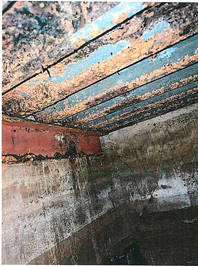
Severe Corrosion of the Metal Pan and Entrance
