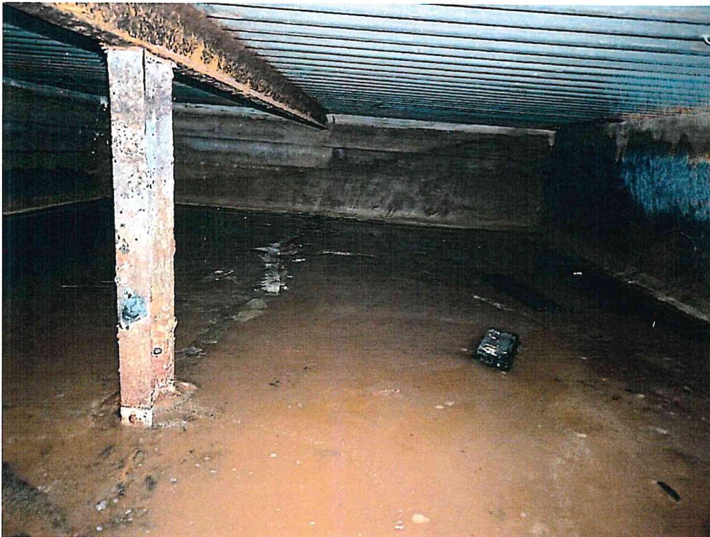
Pan in fair condition – Column and Beam in Poor Condition
