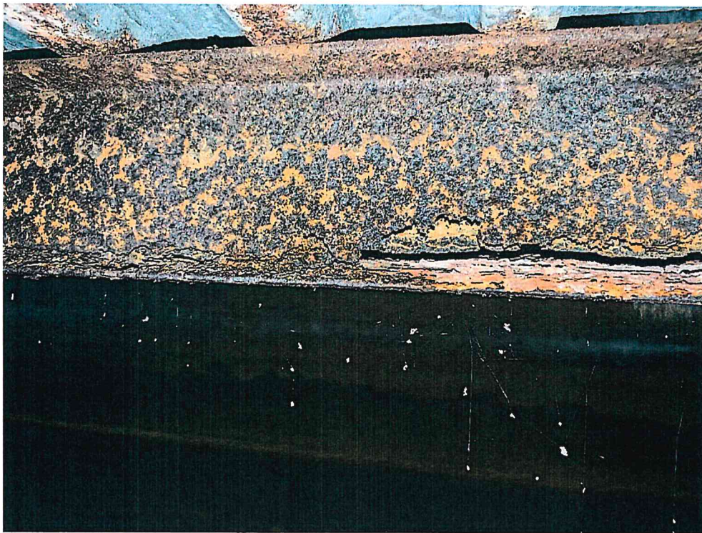
Scaling of the Beam Supporting Metal Pan
