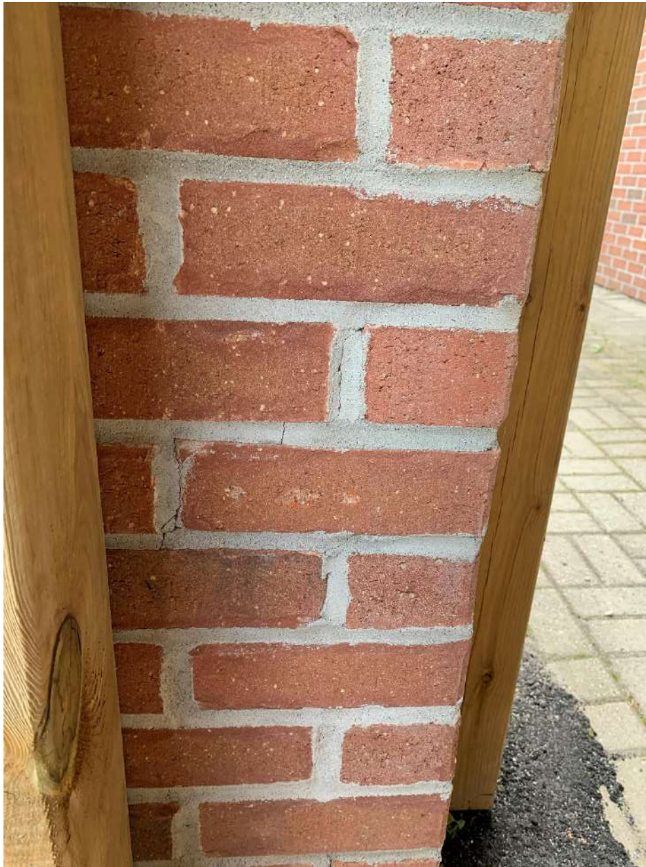
Figure 19: Cracks in brick pier.
