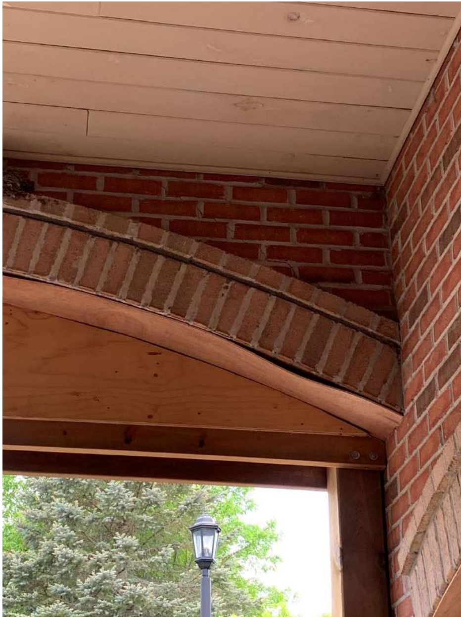
Figure 4: Cracking at top of arch, indicative of improperly installed lintel.
