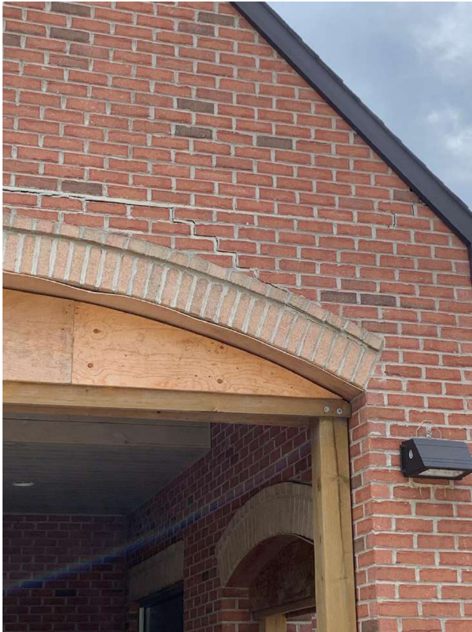
Figure 14: Lintel failure at main arch.
