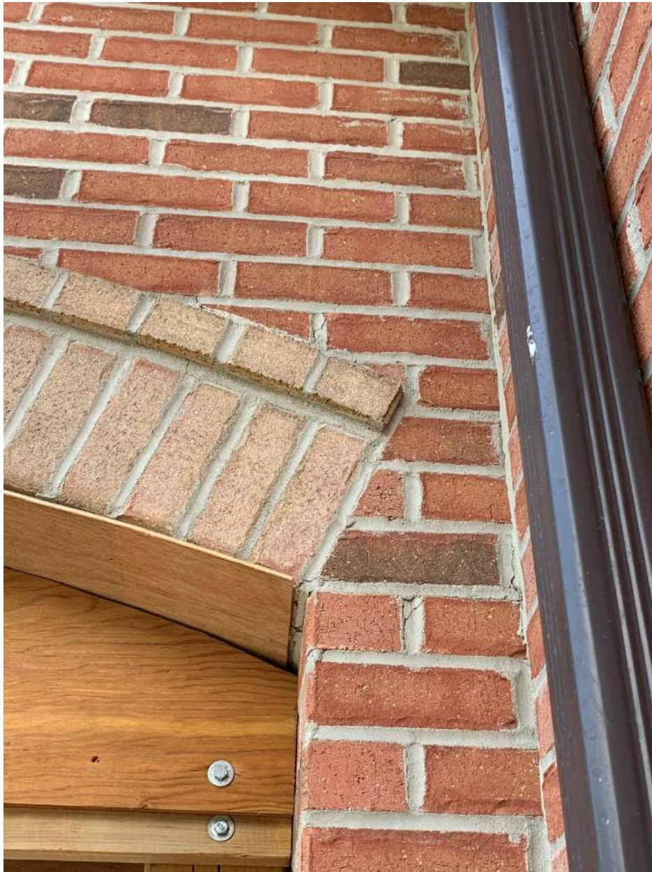
Figure 20: Minor cracks at arch.
