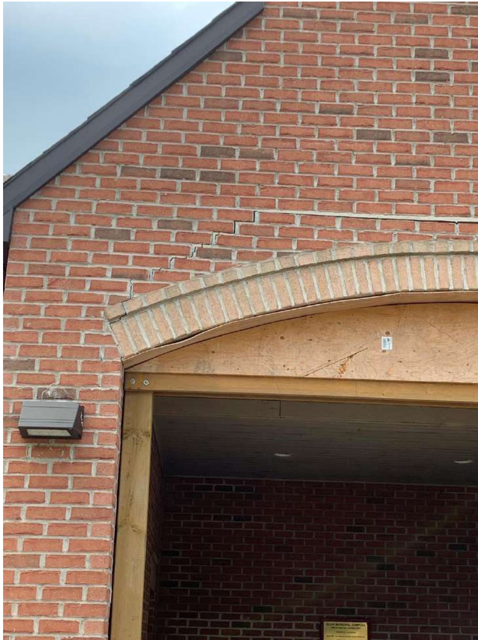
Figure 13: Lintel failure at main arch.
