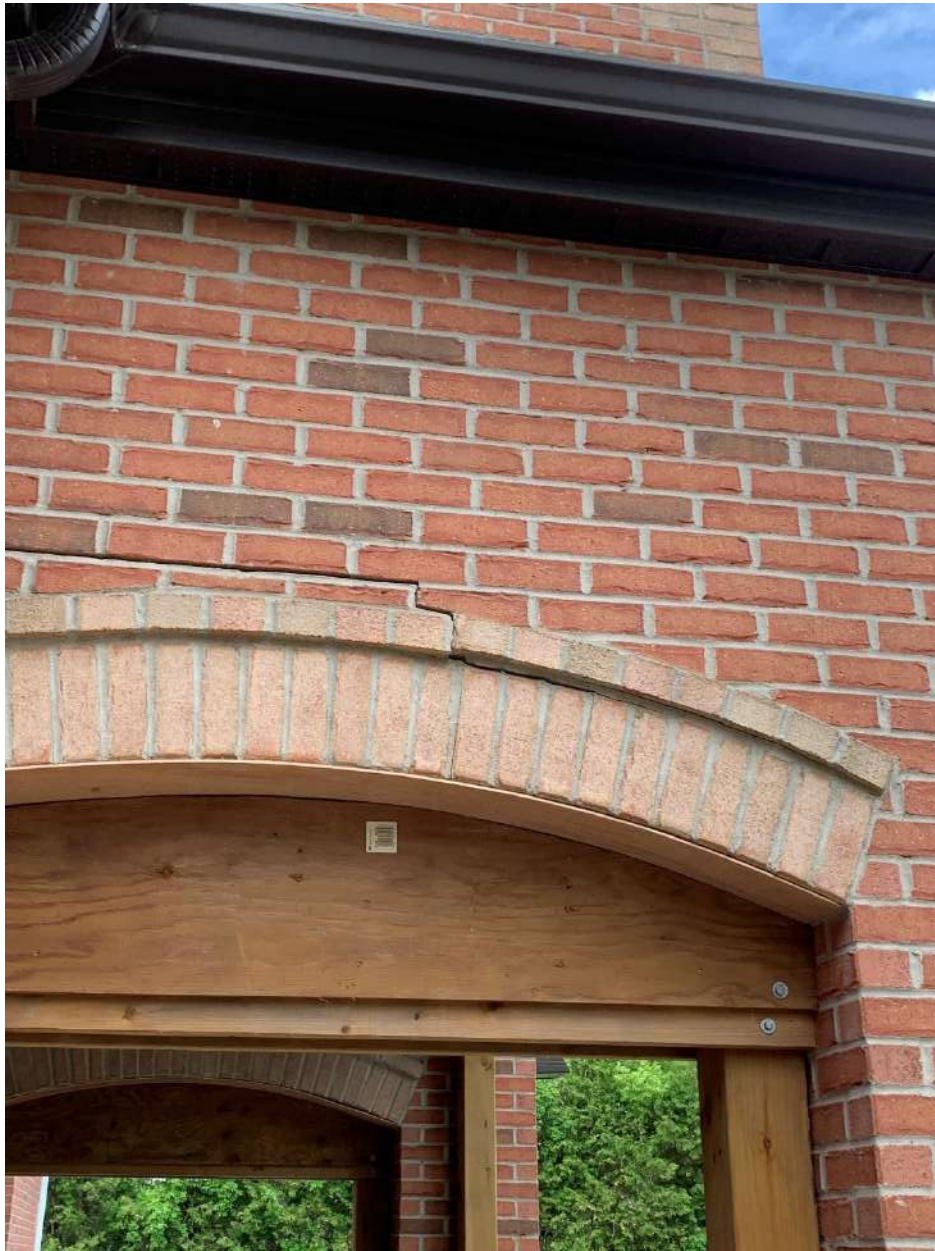
Figure 9: Cracking up to the underside of the assumed location of brick lintel.
