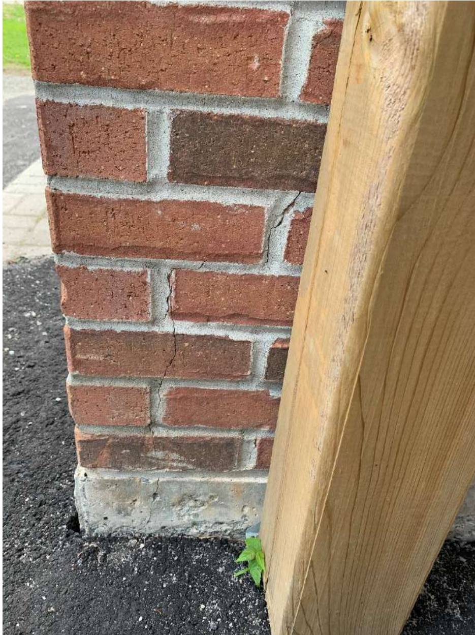
Figure 18: Cracks in brick pier and concrete pier.
