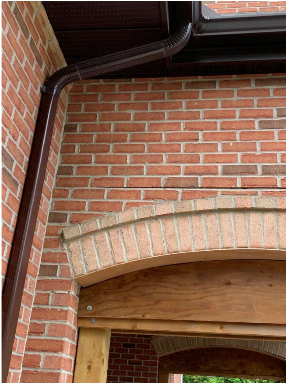
Figure 8: Thicker bed joint on side arch, indication an lintel at this location.
