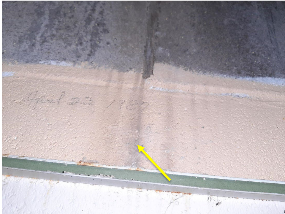
Photo 1 – Mould growth on block wall.
