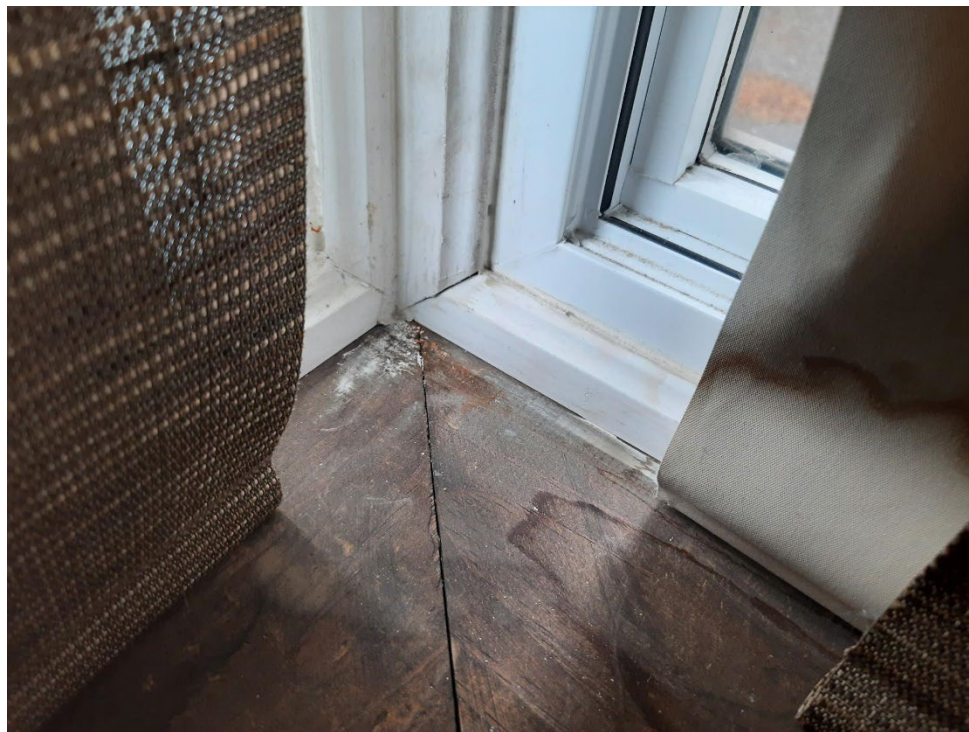
Photo 4 – Water staining on window sill.
