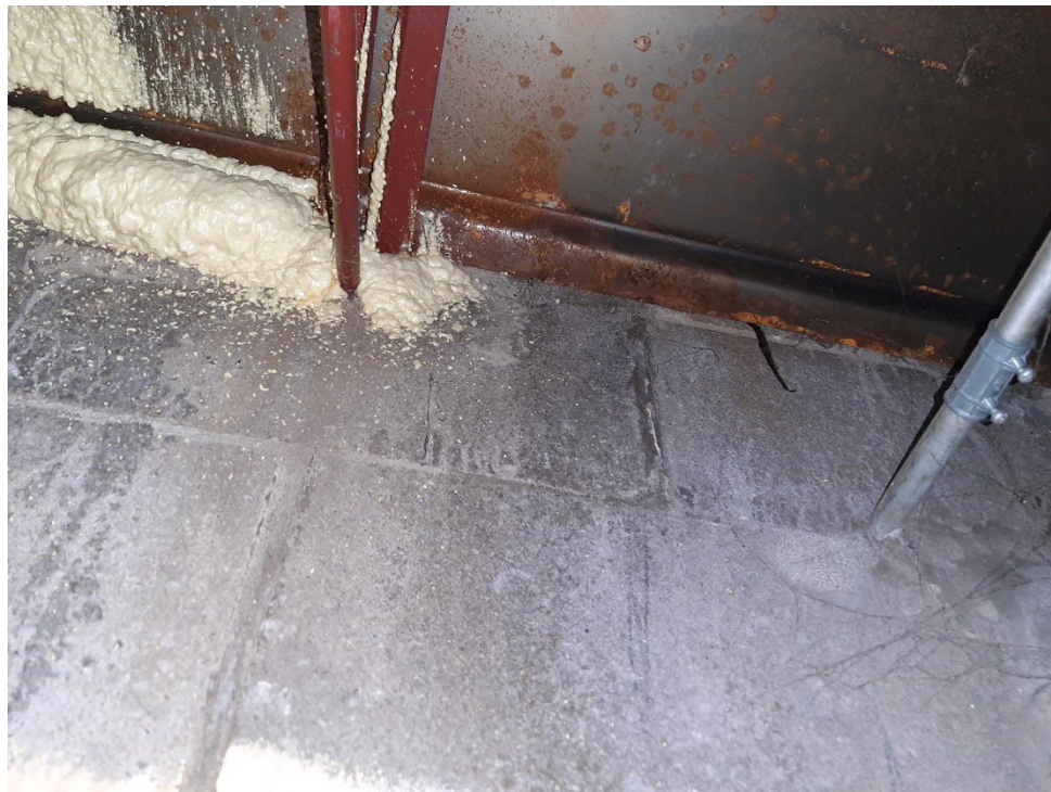
Photo 2 – Mould growth on block wall.
